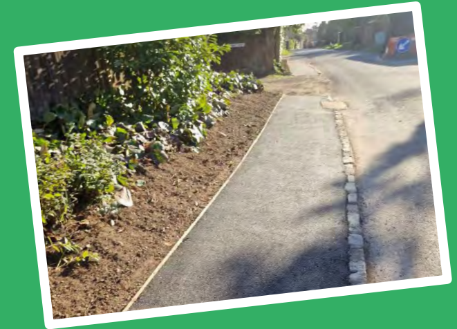
Footway on Blackpond Lane
